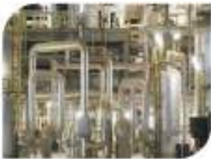
Water Piping System
